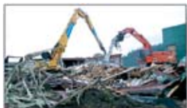
The Winfrith fuel fabrication facility during operation, and then during demolition of the decontaminated building shell, United Kingdom.
