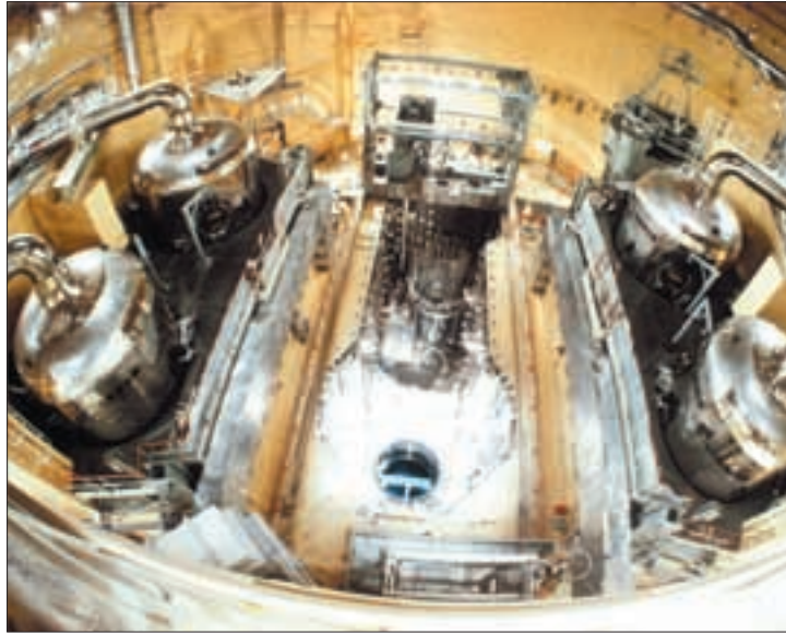
The reactor vessel and four steam generators at the Tsuruga nuclear power plant, Japan.
