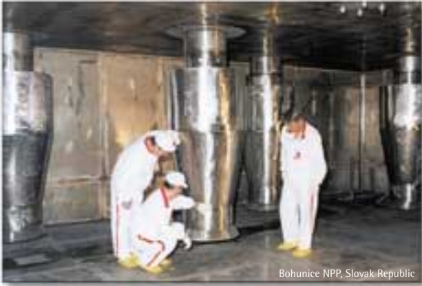
Bubbler condensers at the Bohunice nuclear power plant, Slovak Republic.
