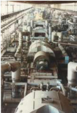
Turbine hall of Greifswald NPPs
