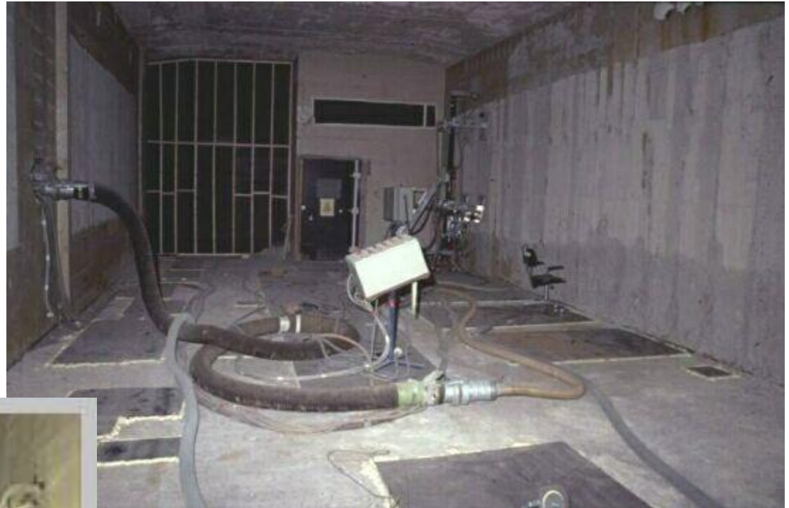
Use on a reprocessing cell wall
