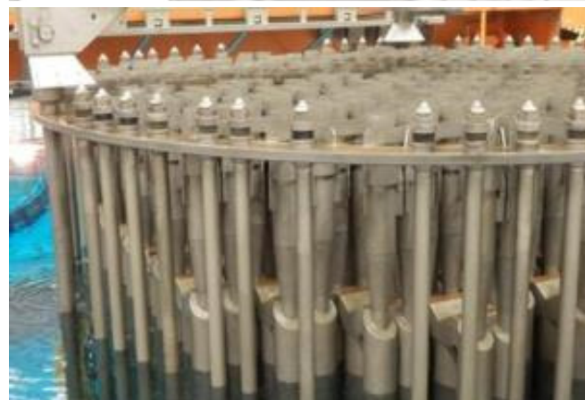
WATER SEPARATOR ABOVE WATER LEVEL AFTER FSD (2015)
