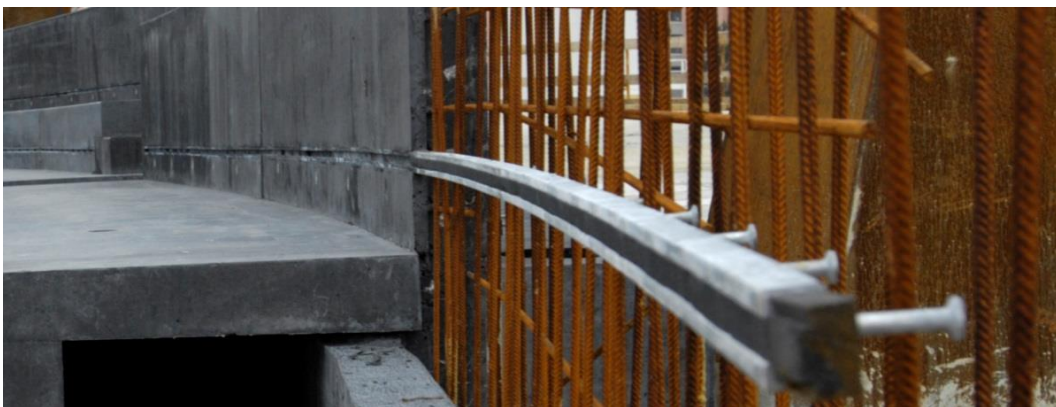
Figure 3: Anchor rails in a conventional building showing the link to the reinforcement steel [4]
