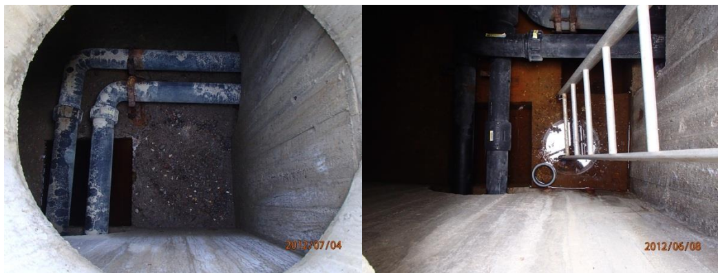
Figure 4. Well shaft in two manholes in non-viable part of the active pipes (with and without ladder).
